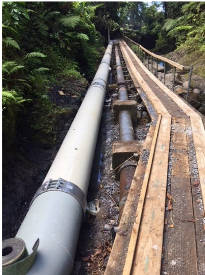
Most of the GRP used for the two schemes was placed underground, except in areas where a trench could not be dug.
